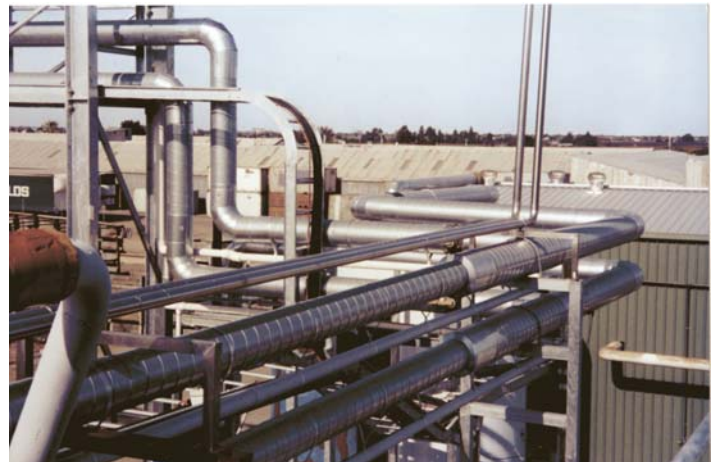
Refrigerant lines supported from outer casing - no vapour barrier penetrations, no sweating and no ice ups.
