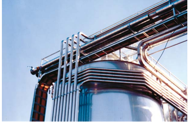
Refrigeration pipelines outdoors in Queensland - under budget and on time.
