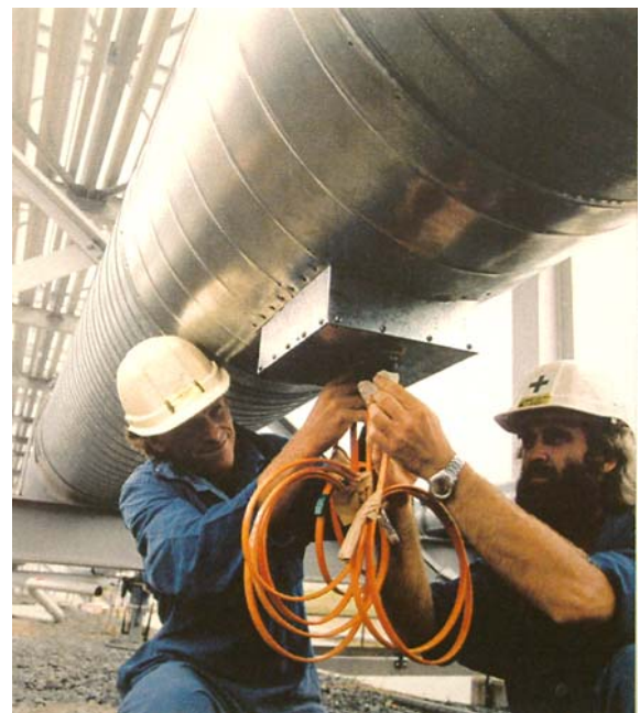
■ HCU Feedstock - simple system in critical application
