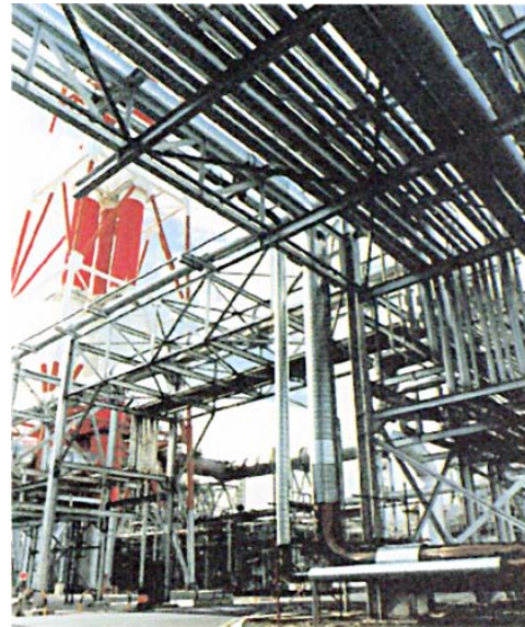
■ Insapipe for hydro cracker feed stock, 2.5km long, 600mm nb and 200mm nb at road crossing.
