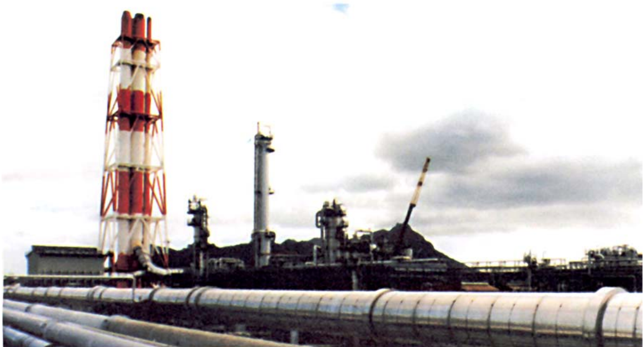
■ Insapipe 600mm nb residue import line, 2.1km long at NZ Refining Company, Marsden Point
